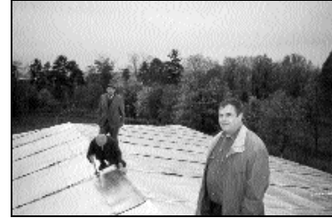
Contractors install a new roof of galvanized steel at the Zaluchya orphanage. The roof replacement was made possible by a grant from the Ukrainian Orthodox Church of the USA.
